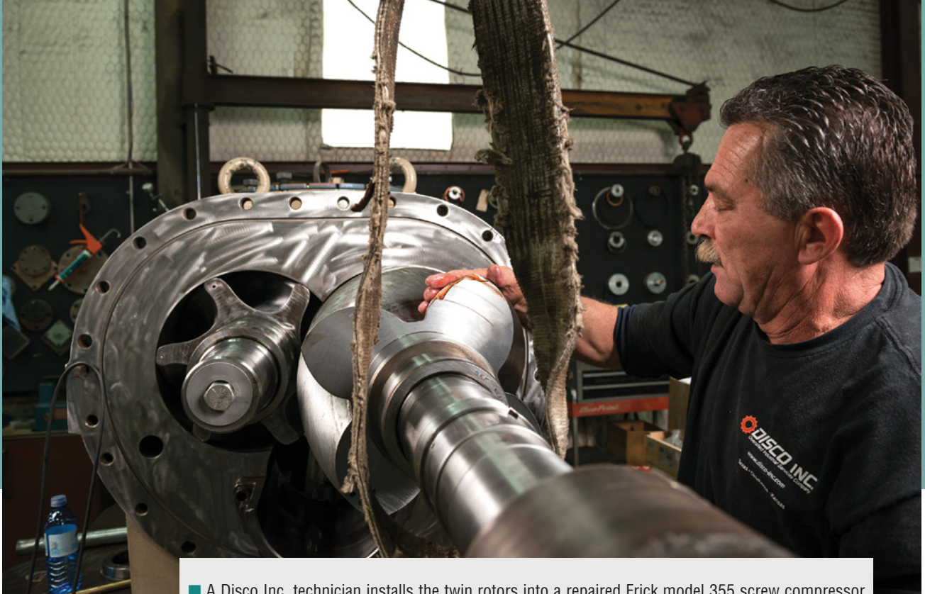
■ A Disco Inc. technician installs the twin rotors into a repaired Frick model 355 screw compressor casing. Disco has been rebuilding screw compressors since 1991, when they were first introduced to the gas fields in the mid-continent area.
